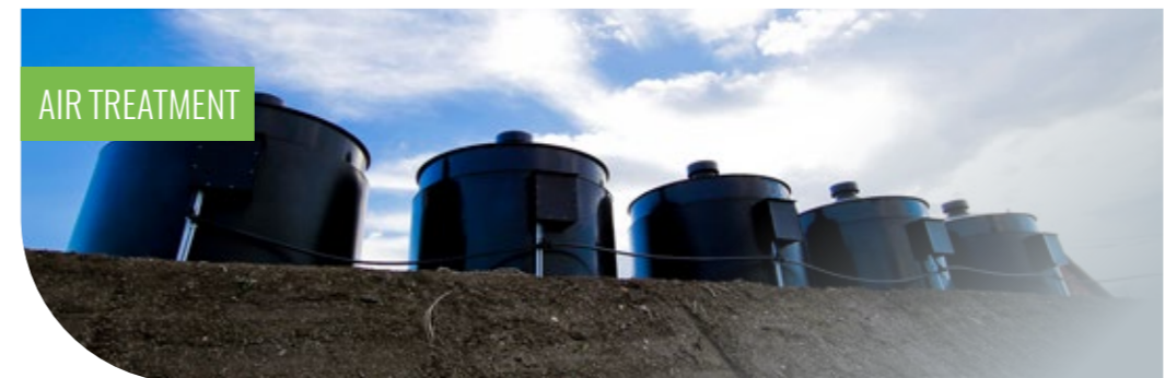
LANDFILL LEACHATE TREATMENT
