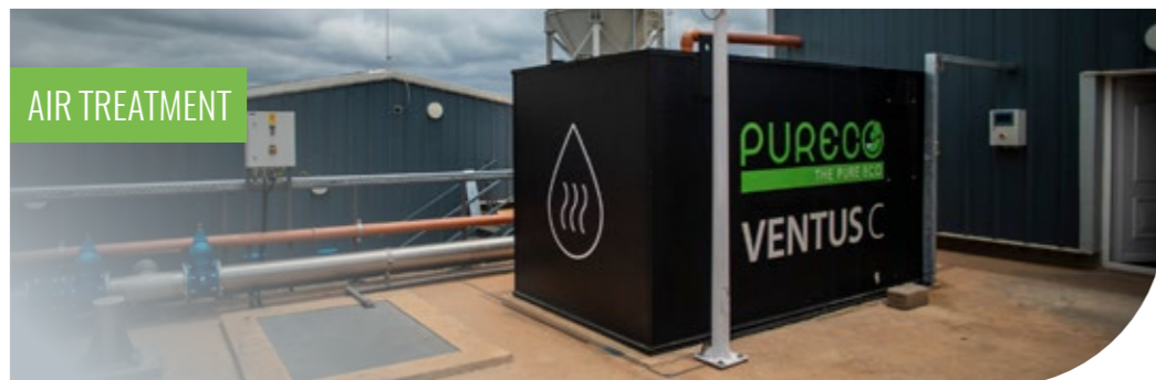
LANDFILL LEACHATE TREATMENT
